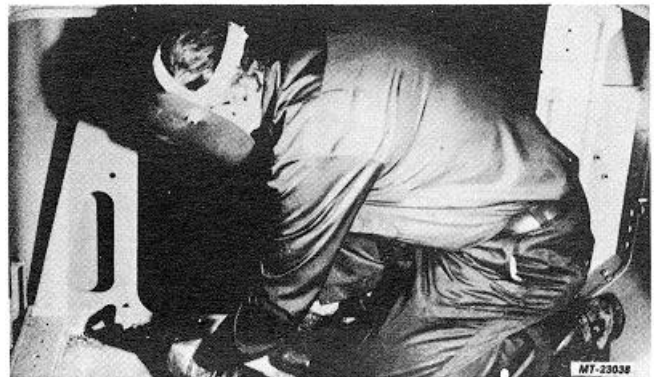
Fig. 49. Seam Weld At Inside Of Side Panel
